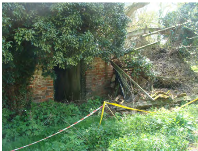
Picture 1.15 Same derelict building, northern elevation. As can be seen southern end is probably incapable of meaningful restoration
