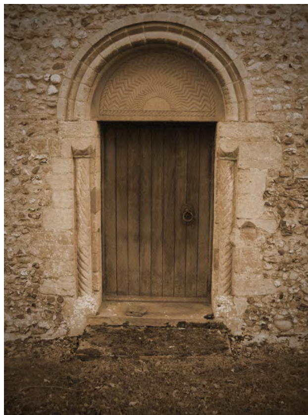
Picture 1.3 North door of St Mary's Church. Flintwork and dressings of Barnack stone
